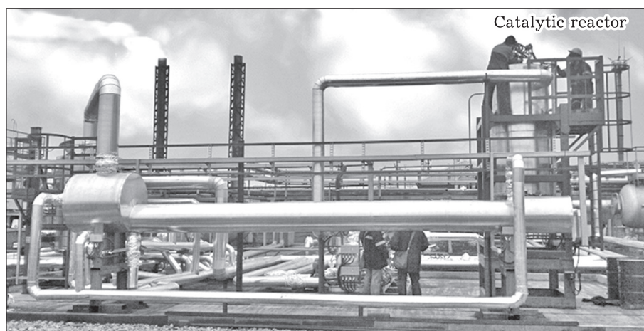
Fig. 4. Appearance of an industrial plant for treatment of associated petroleum gas (APG) using direct catalytic oxidation.
